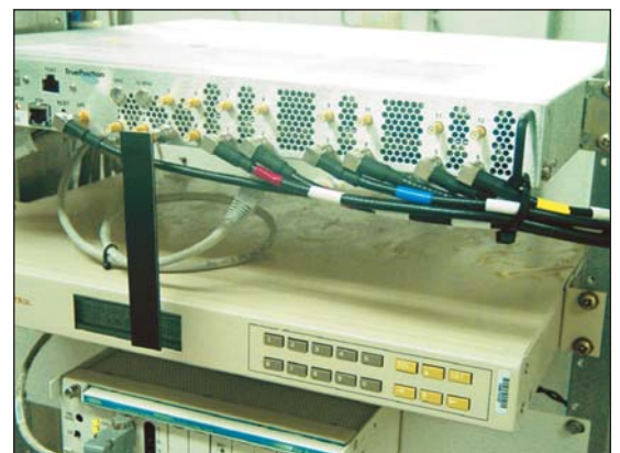
Figure 1 • E911 location determination equipment must be reliably connected to the wireless system equipment.
